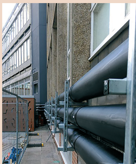
Low diameter plastic pipes have been mounted on the walls of existing buildings to avoid the cost of digging up the roads
