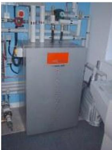
The Heat Pump in the GSHPA offices
