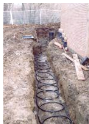
The 'slinky' ground loop being installed in a trench at the National Energy Foundation
